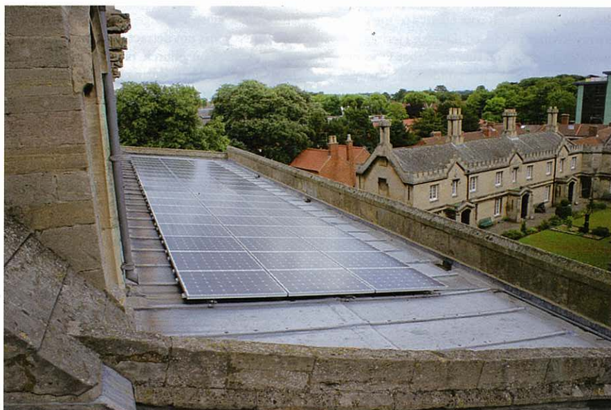
Photo-voltaic panels on the south aisle roof of St Denys' Church, Sleaford (Photo: Julian Patrick)
